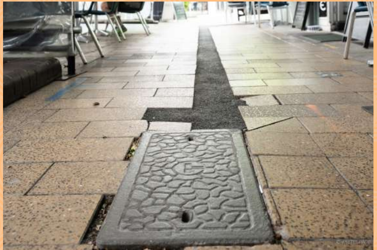
Footpath damage in Marrickville Rd
